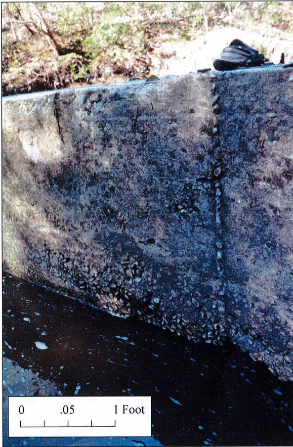
Photograph 7. Detail of Aggregate Concrete
